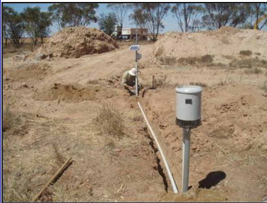
The Hi-Tech rain gauge & monitoring station
